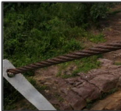
Figure 5: Cross section and image of top wire rope of the handrail
