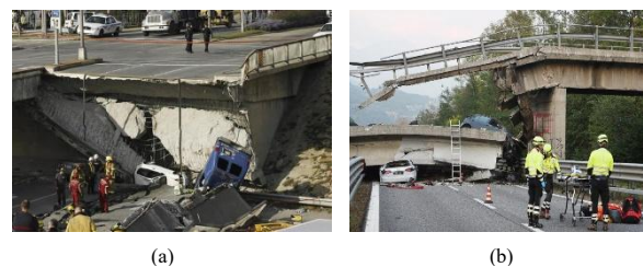
Figure 2 : (a) Concord overpass collapse, Laval, Canada 2006 Overpass collapse; (b) Lecco, Italy 2016
