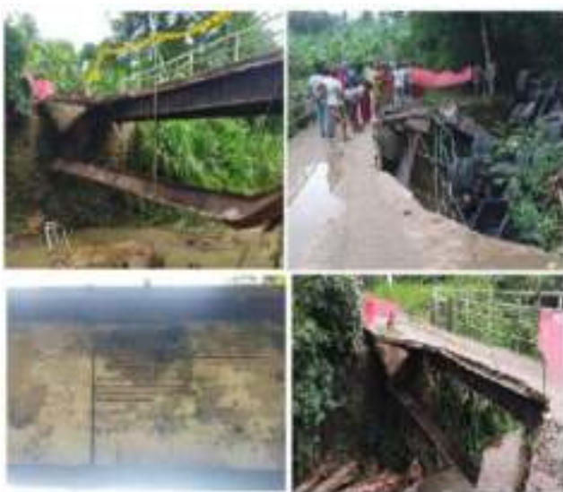
Images taken after the failure of a bridge in Meegahapitiya- Kottagala road in Maddula area
